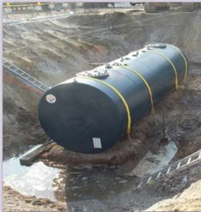
UST with hold down straps on a concrete pad. Credit: EPA
